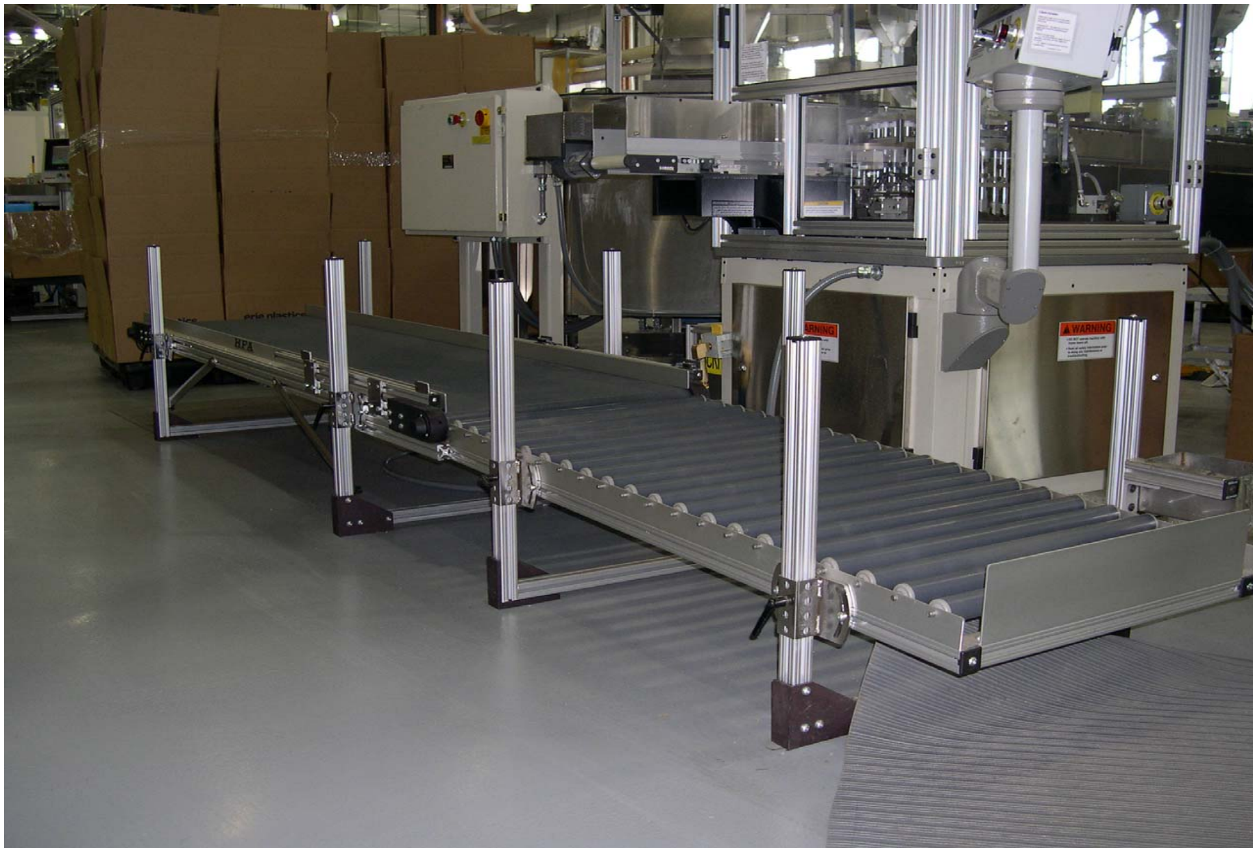
2270 Gravity Roller Attached to Inline Box-Fill System on a Packaging Machine
